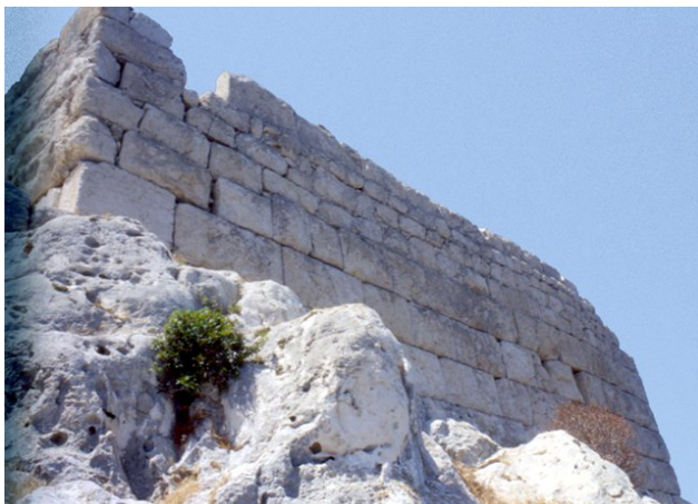
Figure 4. The north facade before the collapse. (KB' EPKA)
