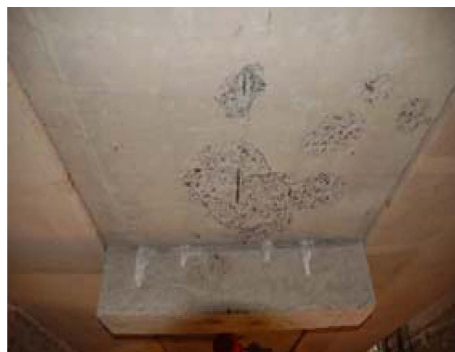
Fig. 5 Spalling on the bottom of slab
