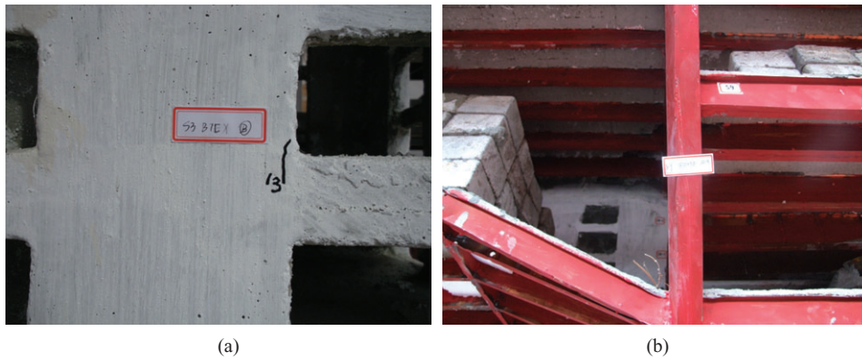
Figure 12. (a) Crack at the end of coupling beam. (b) Slight twist of inclined column.
