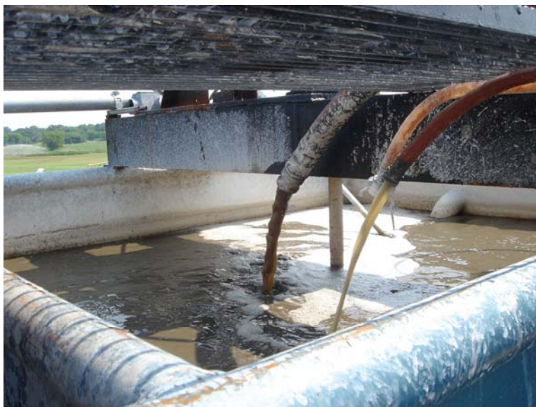
Figure 2. Mixing tank in the Electrocoagulation System
