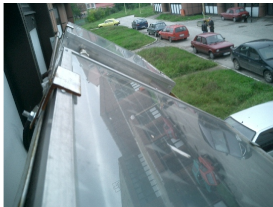
Figure 6. Outdoor part of installation of hybrid solar collectors
