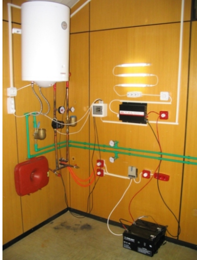
Figure 7. Indoor part of installation for use of hybrid solar collectors
