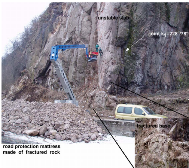
Fig. 7. Detail of the unstable slab and of the fractured rock portion at its base.
