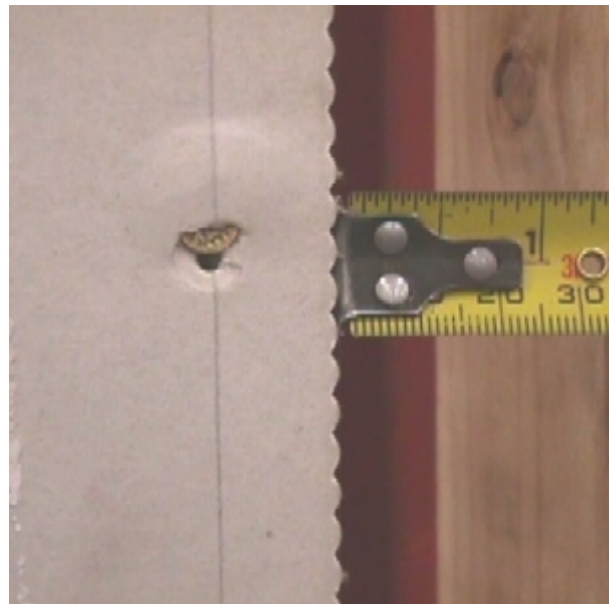
Fig. 5 Typical failure mode of a nail connection between plasterboard and frame in shear. (Note: Tearing of plasterboard and embedment of the nail head within the thickness of the board).
