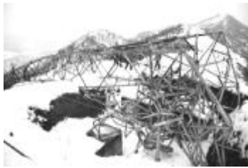
图 1 输电线路由于覆冰严重发生倒塔 Fig. 1 Tower collapsed caused by severe ice-coating of transmission line
