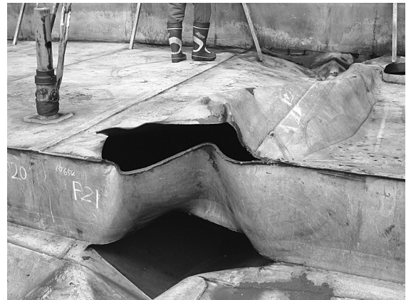
Fig. 6 Failure of pontoon.
