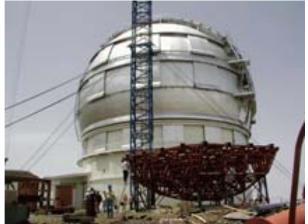
Fig. 3. A view of the GTC dome with the supporting cell of the primary mirror in the foreground, soon to be integrated in the telescope structure.
