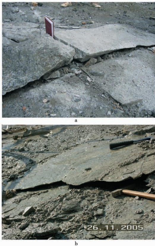
图1 坝基开挖岩体岩爆和张性剪切破裂现象 Fig. 1 Phenomena of rock burst and tension-shear failure in dam site excavation
