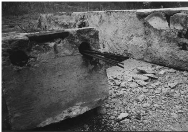
Fig 12. Rupture of bridge staircases due to corrosion of prestressed tendons
