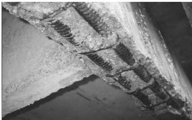
Fig 5. Debonding and corrosion of longitudinal bars and stirrups of reinforced concrete bridge beam
