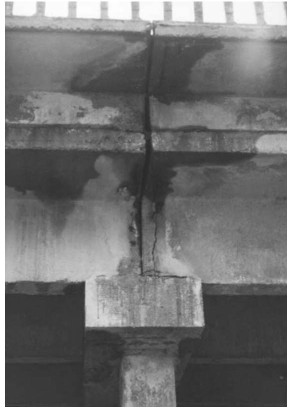
Fig 9. Deterioration of edges of beams and cap of pier due to leakage of expansion joint
