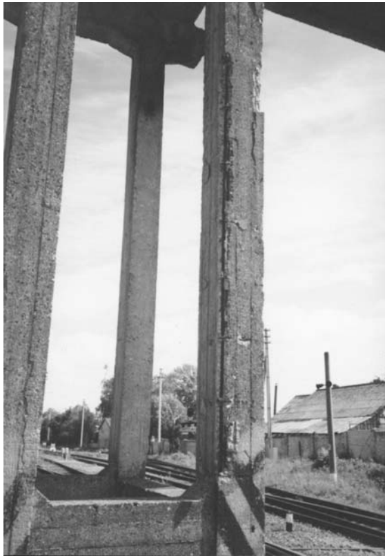
Fig 4. Corrosion of reinforcement of the multiple-column pier accompanied by cracking and deterioration of concrete cover
