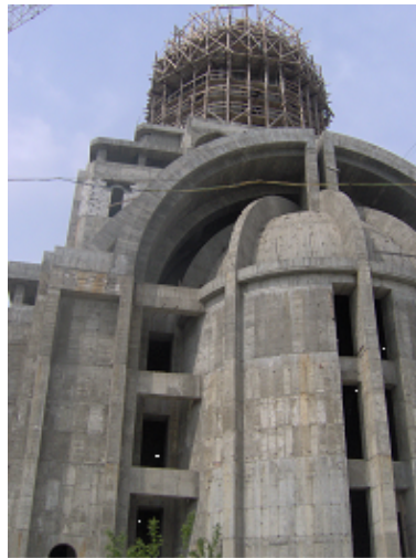
Fig. 1. – Cathedral's dome from where rain infiltrates in the Civil Defense Shelter.
