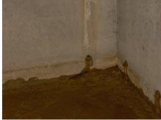
Fig. 3. – Seepage through the metallic sheaths.
