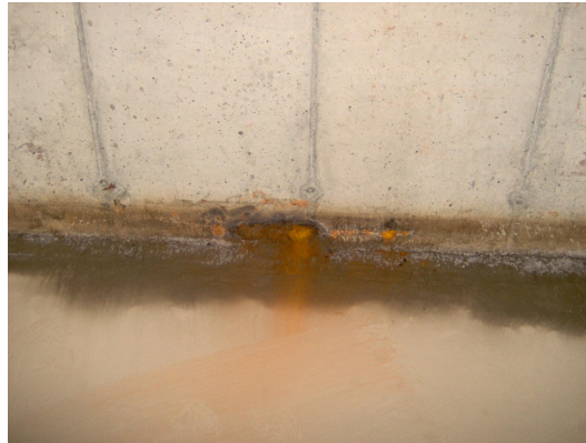
Fig. 2. – Massive seepage in the Civil Defense Shelter through the metallic sheaths of formworks.
