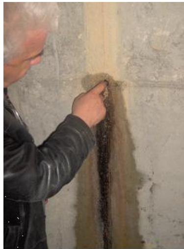
Fig. 4. – Seepage with sediments from metallic sheaths.
