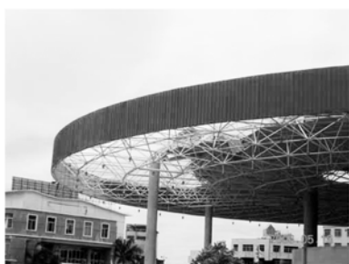
图1 圆形罩棚式建筑屋面围护结构破坏 Fig.1 Damage of envelope structure on circular canopy roof building
