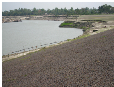
(a) Erosional point at Bhuiyapur (bend scour developed around the bridge abutment).
