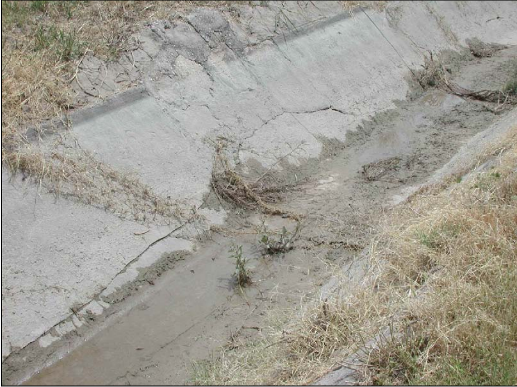
Figure 7. Horizontal cracks in the sidewall of MA4.
