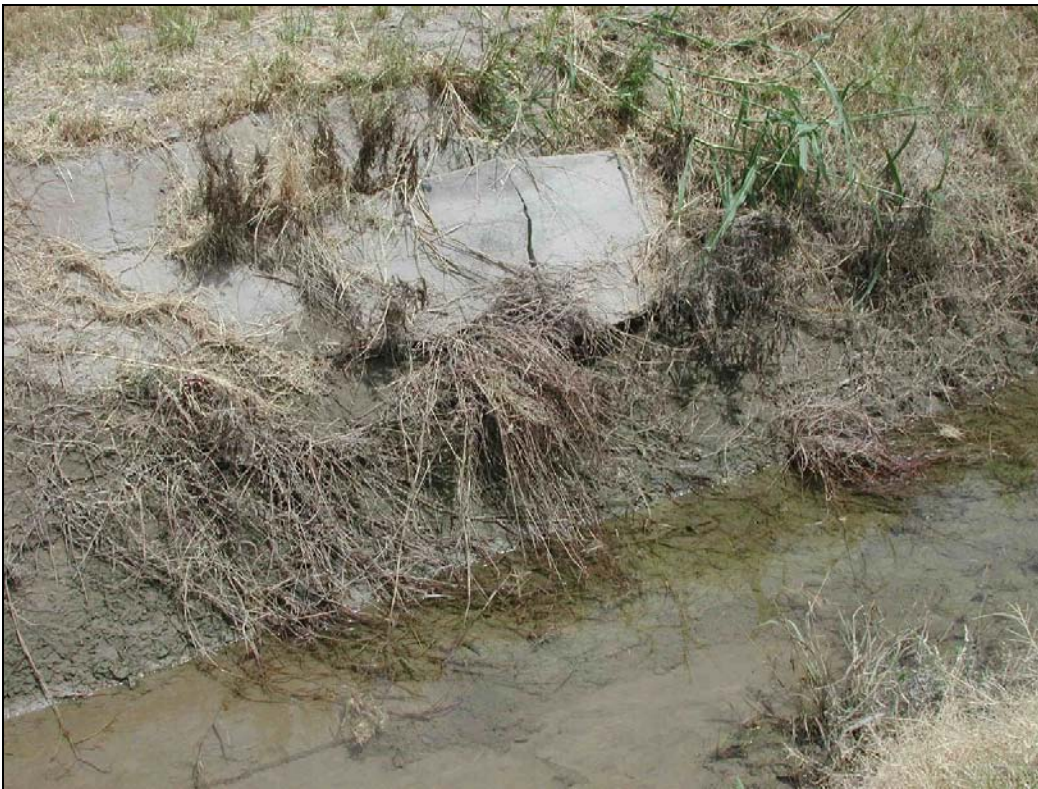
Figure 8. Large break in the sidewall of MA4.
