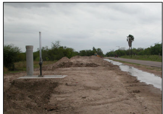
Figure 2. Visible leaks shown after construction
