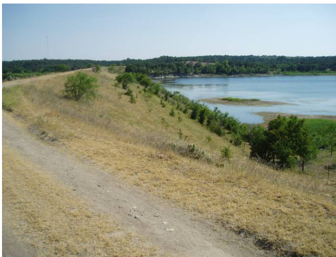
Figure 1. PL566 structure in the Bosque watershed with sediment build-up and brush growing on the dam
