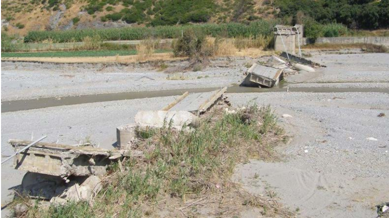
Figure 1: Example of failed bridge due to scour
