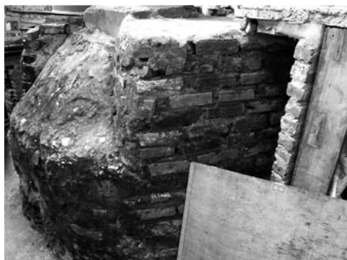
Fig. 18(c) Ruin of Wall at Position (9)
