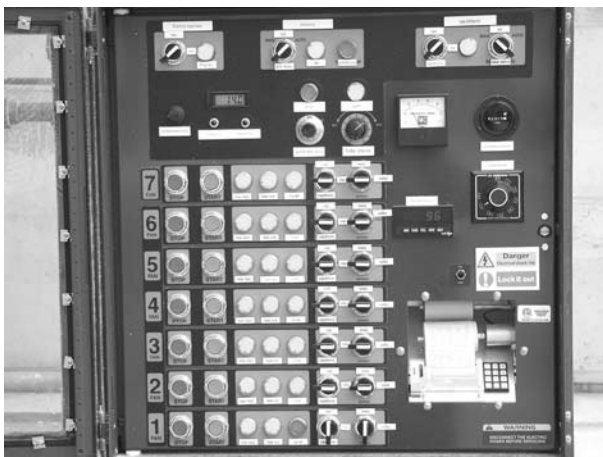
Figure 3. Controlling console of the dryer 1–7 – regulation of fans and burners
