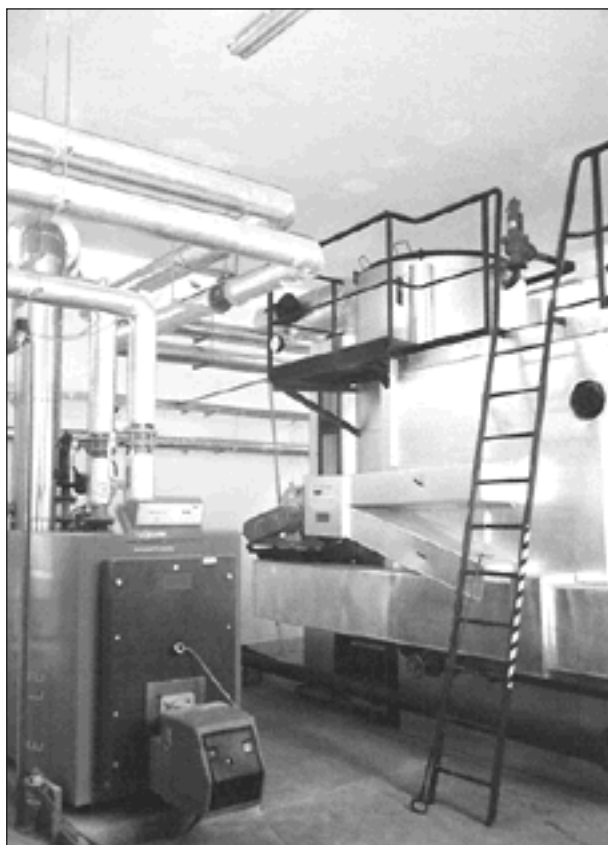
Fig. 2. Boiler TFS 1000 for straw combustion (in the right). In the left side of the picture is reserve heating source Paromat simplex for Biodiesel combustion
