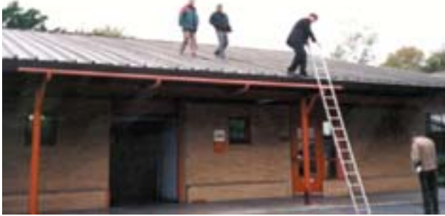
Labour inspector stopping dangerous work at height
