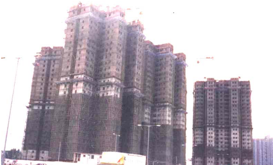
Figure 4.2 Double layered scaffold
