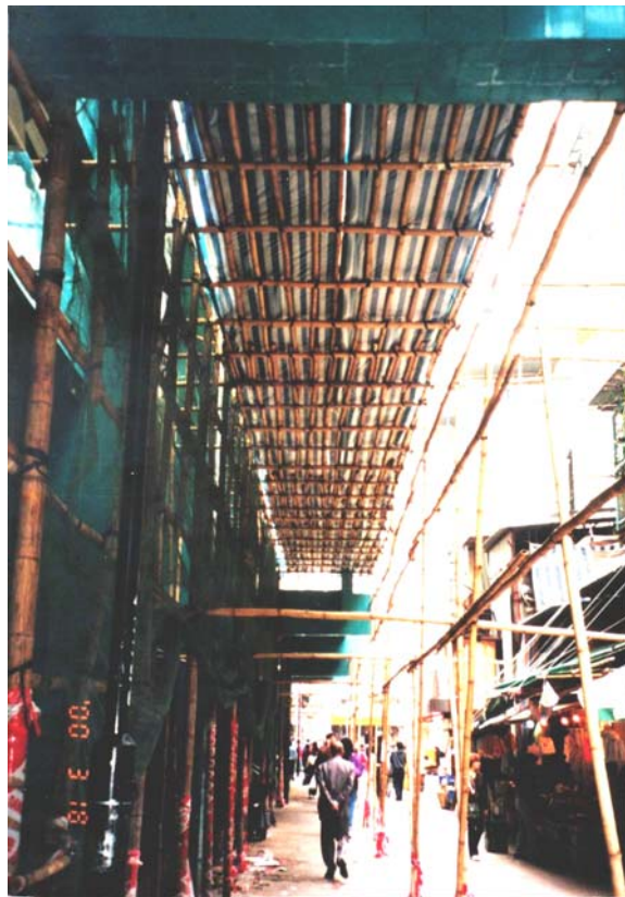
Figure 4.4 Obstruct plate in double layered scaffold
