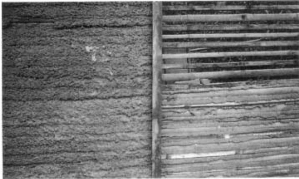
Fig. 18: Mounted paneling partially covered with cement/sand mixture
