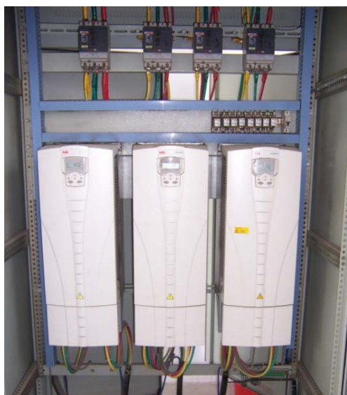
Figure 6. Frequency conversion power counter 图 6. 变频动力柜
