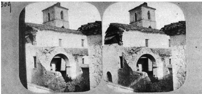
Fig. 6. Damage to the Church of St. Angelo della Trinità according to the Mallet's report (Mallet, 1862, stereoscopic photo no. 309).
