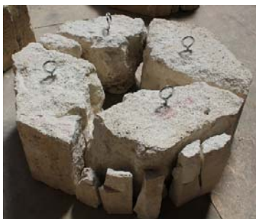
Figure 13. Pillar n. 11 – row I. It is evident the external deterioration of the stone, in good condition in the inner part.
