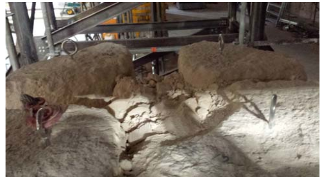
Figure 8. Top images of a pillar during the disassemble step; in the centre, the irregular mortar core of the column.
