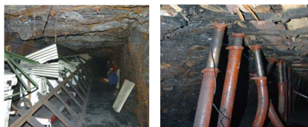
(a) 锚杆索破断
